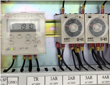
The Group has installed automatic lighting control systems in the new offices in International Finance Centre and Wong Chuk Hang Photo (1)
